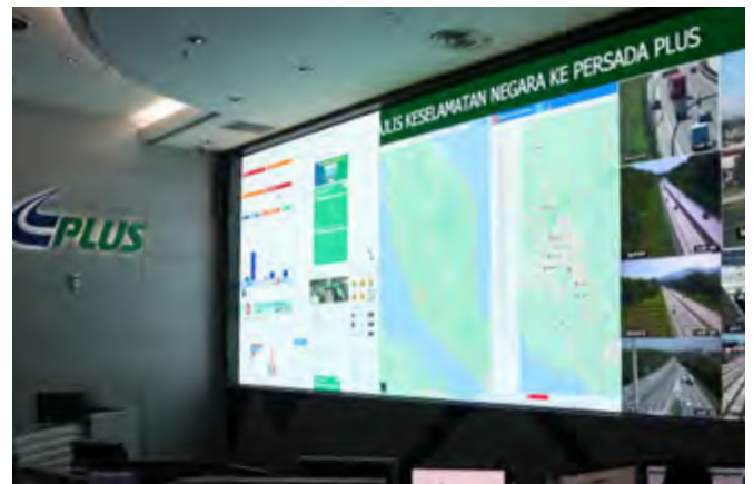
A display of real-time videos and applications to facilitate traffic management on the smart video wall at our TMC.
