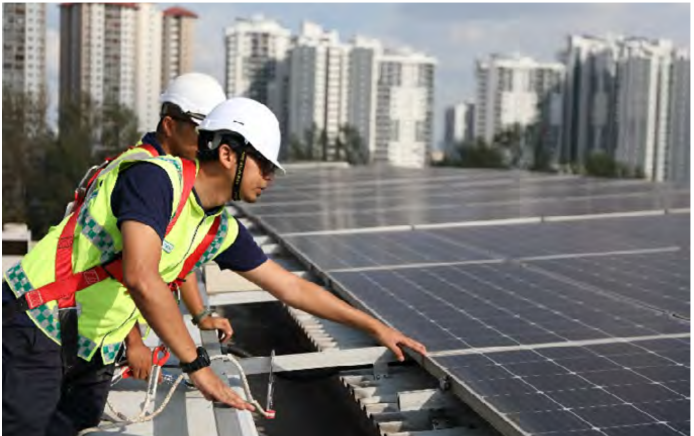
Warga PLUS performing routine inspection on a solar PV system.
