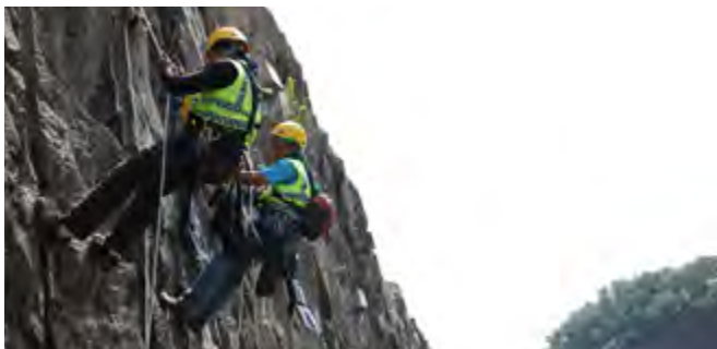
Our maintenance team conducting slope inspection work to ensure the safety of our highway customers.
