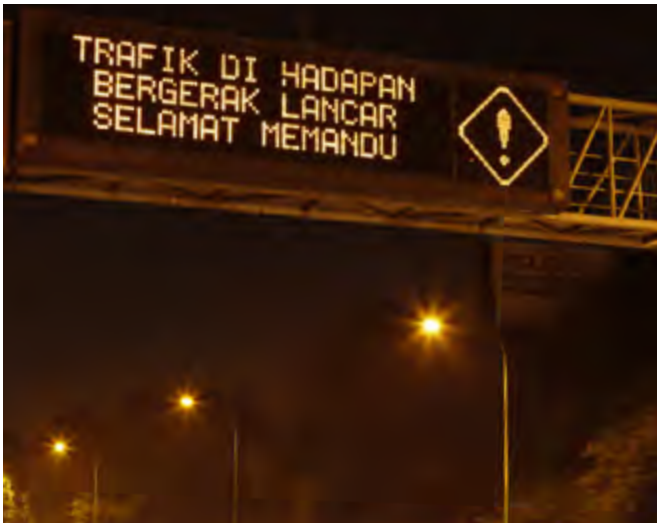
Our VMS displaying traffic updates along one of our highways.
